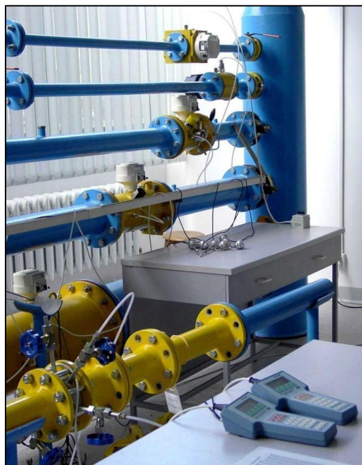
Figure 4.7: Low-pressure air facility.
