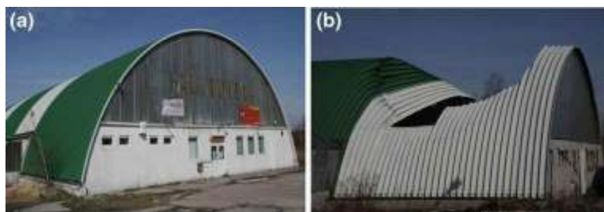
Fig. 1 Examples of a structure (a) in good condition, (b) after failure
